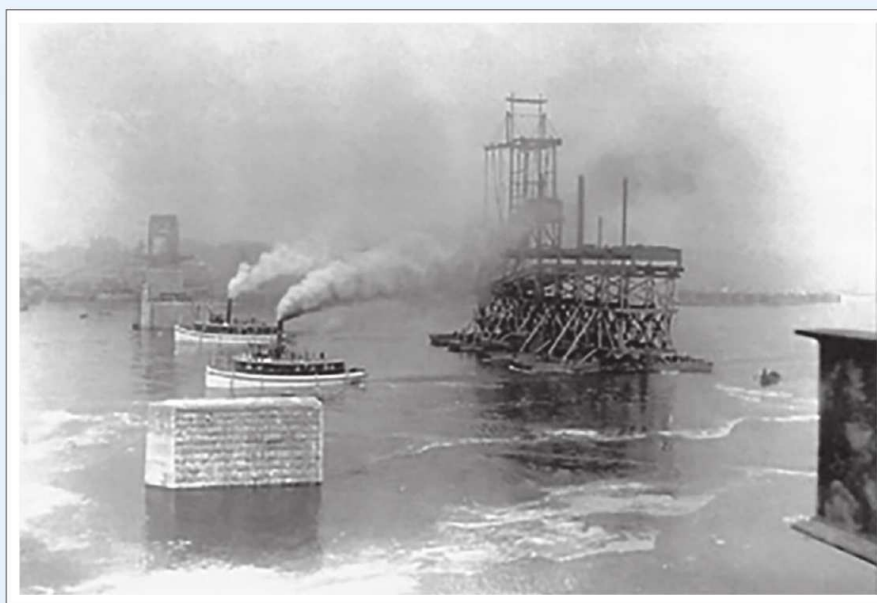
Moving the Anchor Span: Ottawa Transportation Co. tugs Florence and Dolphin tow the anchor span across the Ottawa River on April 21, 1900. The horizontal roadway and sloping bottom chord are clearly visible, as is the erection traveler.
