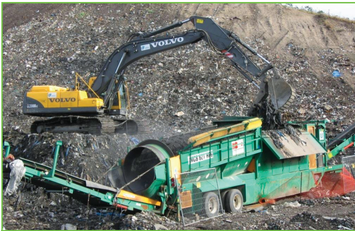
Figure 1C - Excavating most of a landfill to re-engineer the site with a proper base barrier system (Dewaele et al. 2011)
