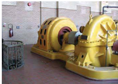
Pumping station interior.
