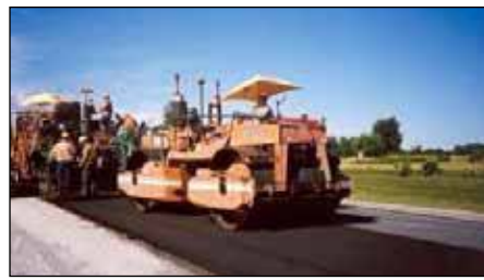
FIGURE 3B: Cold-In-Place Recycling with Expanded Asphalt (CIREAM). Placing and compacting of CIREAM (Lane 2011).
