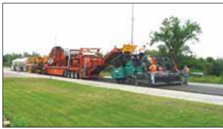
FIGURE 3A: Cold-In-Place Recycling with Expanded Asphalt (CIREAM). CIREAM train (Lane and Kazmierowski 2005b).
