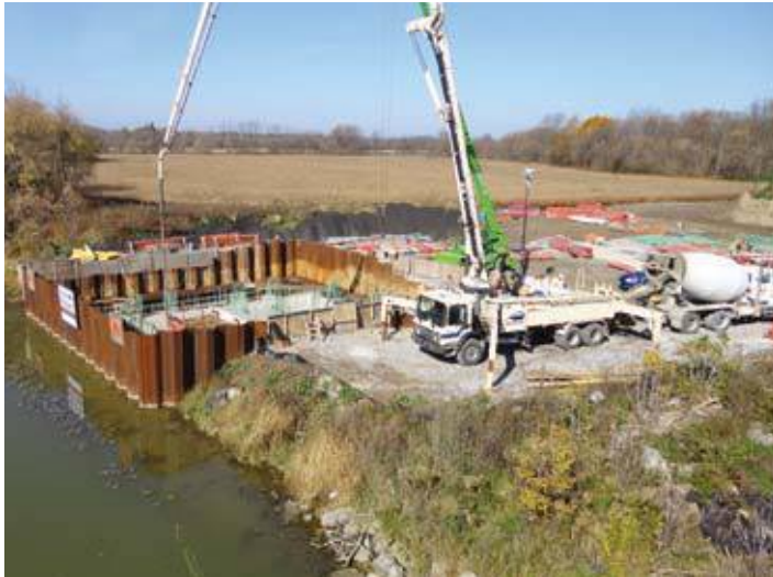
Construction of multi-port intake structure along the Grand River; there are also two twinned below-grade conduits to store raw water in case of contamination occurring upstream.
