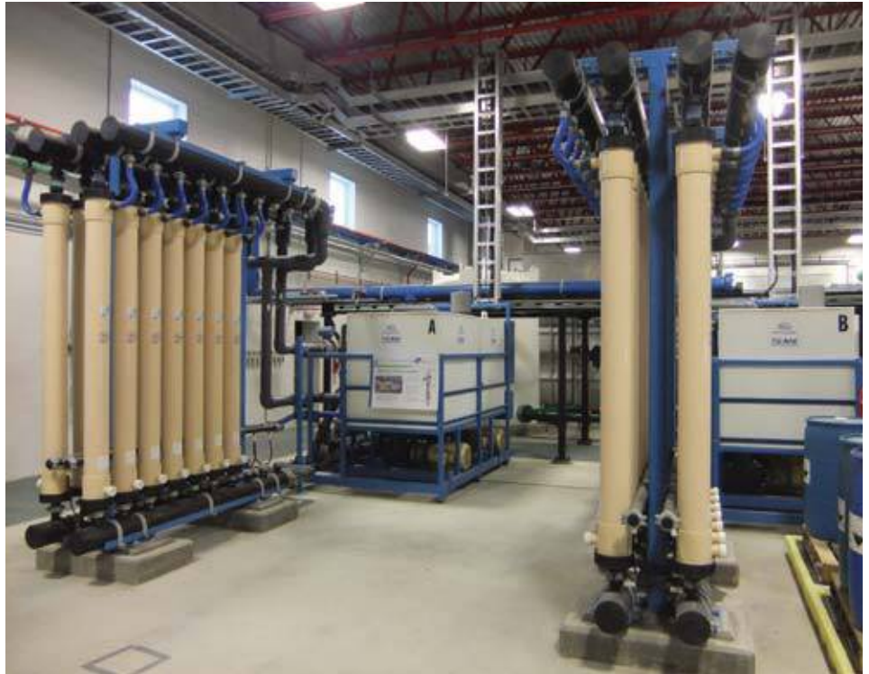
Micro filtration membrane equipment inside the plant.
