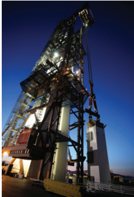
KCB designed the frame to assemble the main tower as well as other structures.
