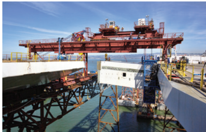
Placing the first of 19 cross-beams that connect the two orthotropic box girders. The temporary works required 25,000 tonnes of structural steel, more than the original Oakland Bay Bridge.
