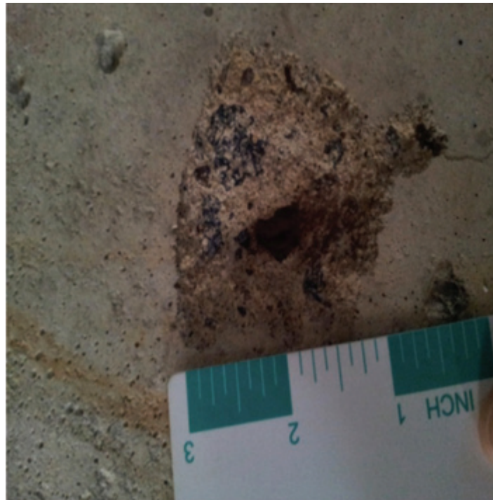
Figure 3: Oxidation of an aggregate particle resulting in popout or delamination of the mortar above the aggregate particle.
