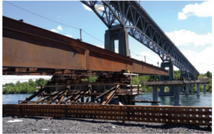
The lightweight launching nose has a sloped bottom chord to allow the girders to land on the piers without the use of lifting equipment.
