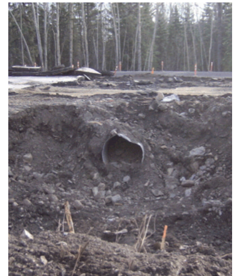
Figure 5: Damage from the 2011 floods in B.C. Photo: Bill Cheung
