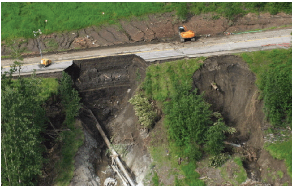
Figure 4: Damage from the 2011 floods in B.C. Photo: Bill Cheung.
