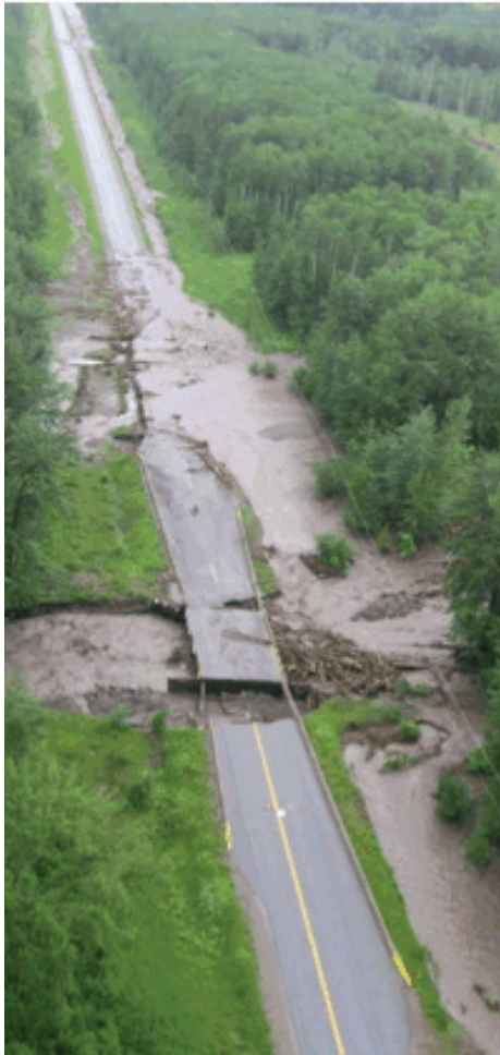
Figure 6: Logs and bedload quickly created dam-like pileups in B.C.'s 2011 floods.
