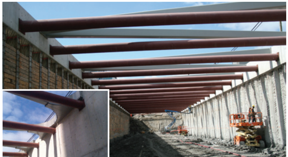
Permanent painted struts will appear as tear drops when seen from above. Temporary unpainted struts provide further lateral support to the centre pile and lagging wall.
