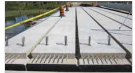
FIGURE 8: View of the Adjacent Box Girders used in Sunshine Creek Bridge Hwy 11/17 built in Summer 2007 (courtesy of Pultrall-Trancels Inc.).
