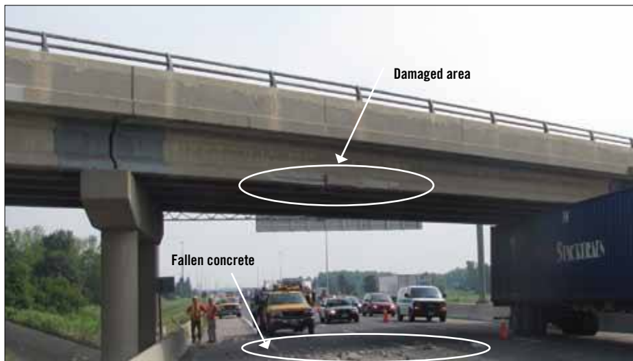
FIGURE 5: Damage to the Dingman Drive Bridge.
