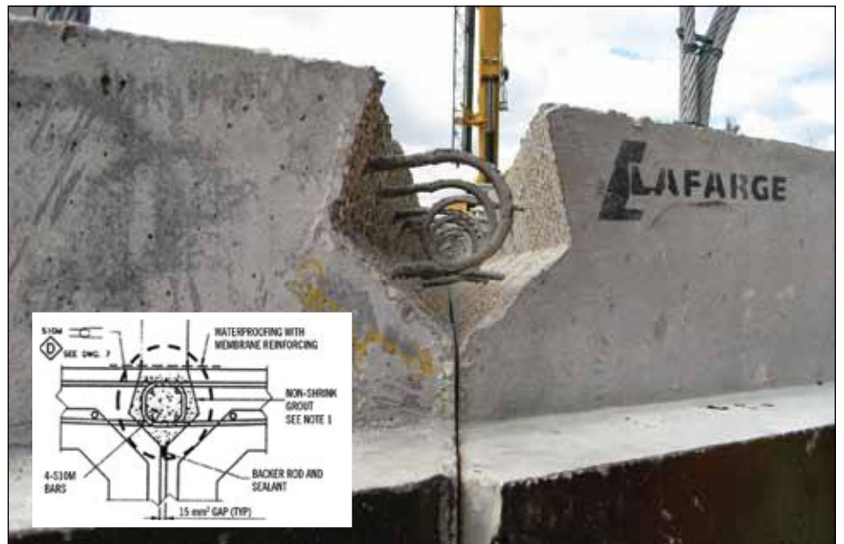
FIGURE 9: Close-up View of the Closure-strip between the Top Portion of Two Adjacent Box Girders in Sunshine Creek Bridge (courtesy of Pultrall-Trancels Inc.).
