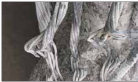
FIGURE 6: Collision-damaged Strands on the Outer Girder.
