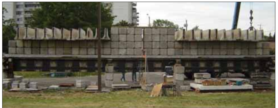
FIGURE 4: View of the Rehabilitated Girder after Loading it with 1368 kN Concrete Weights.
