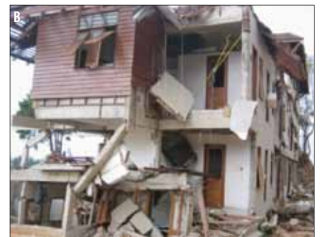
FIGURE 1: Tsunami-related structural damage: (a) Pelluhue, Chile; (b) Phuket, Thailand (Nistor et al. 2009).
