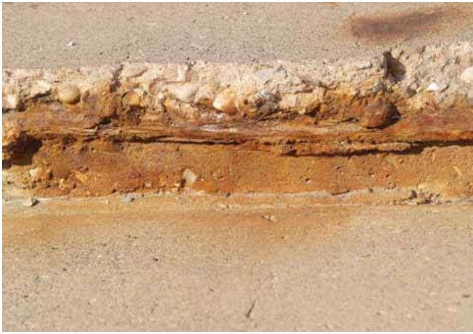
ABOVE: Exposed reinforcing steel in recent (< 15 years) concrete.
