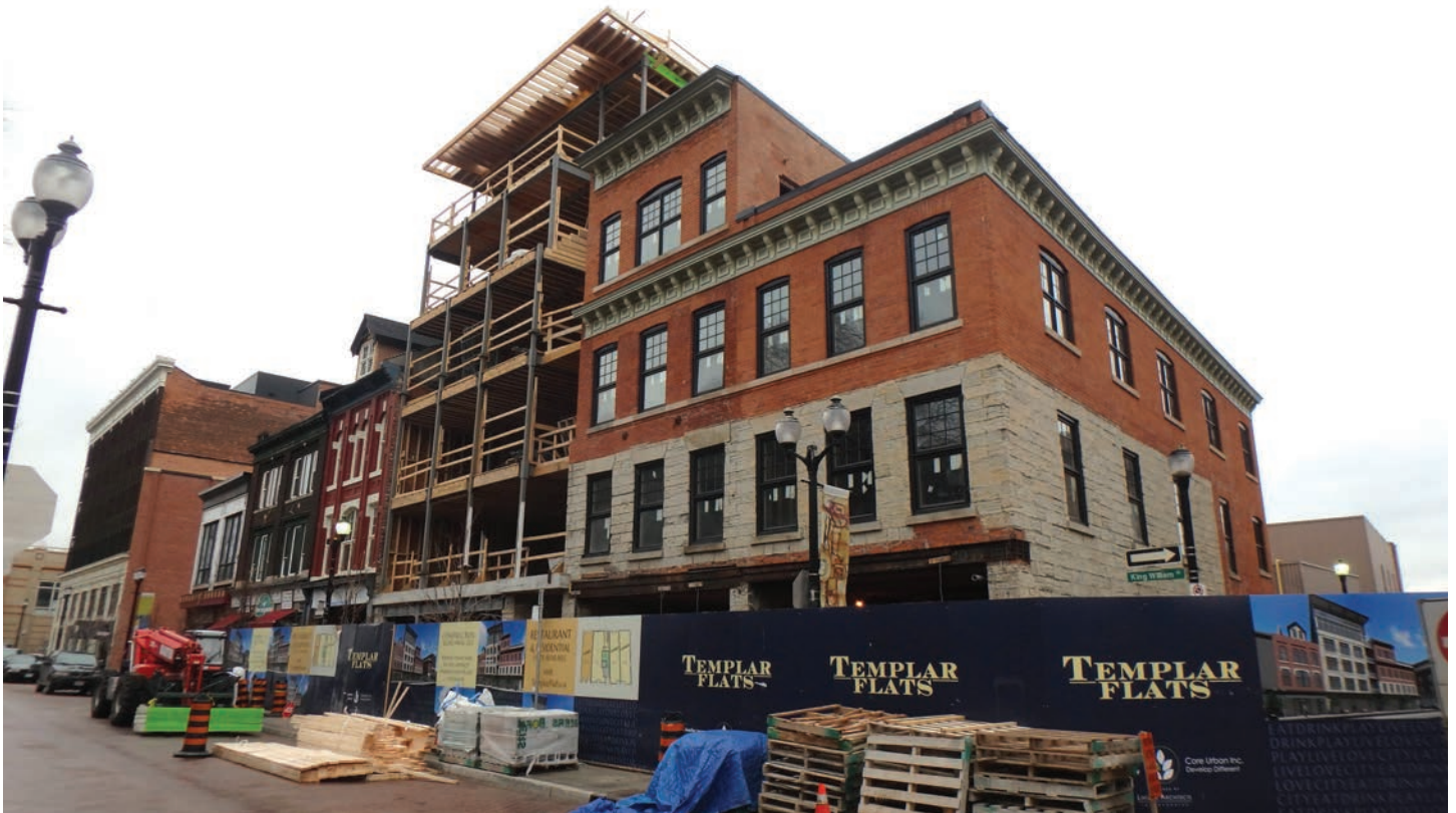
Templar Flats in Hamilton, the first six-story light-framed wood building built in Ontario.
