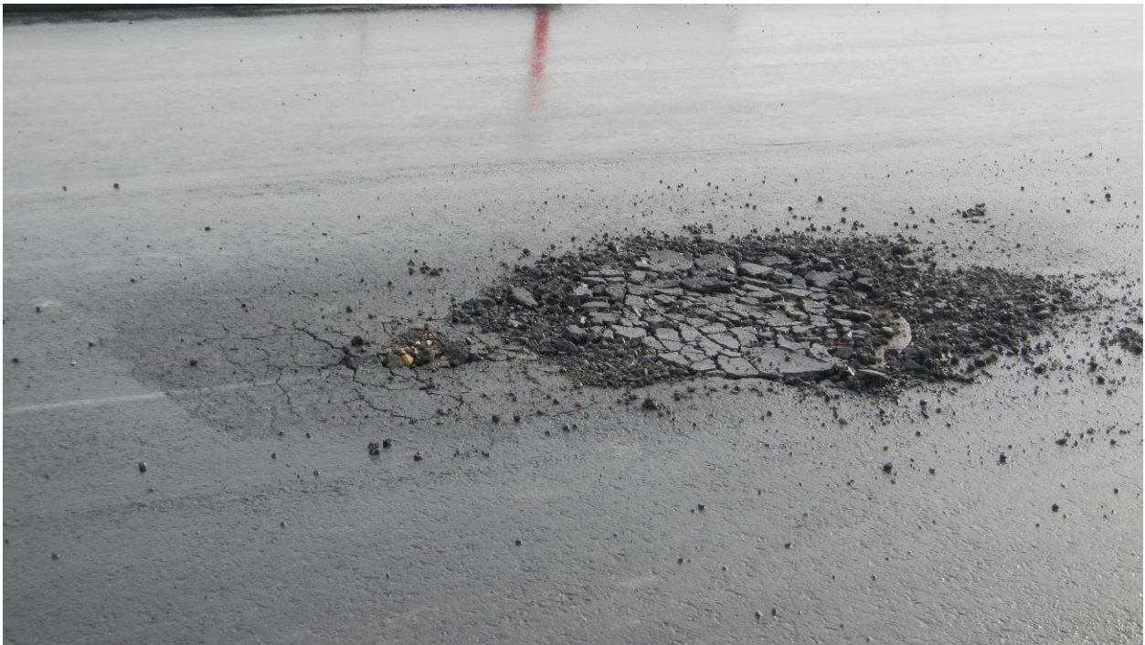
Figure 5: Failure of a Newly Resurfaced Pavement
