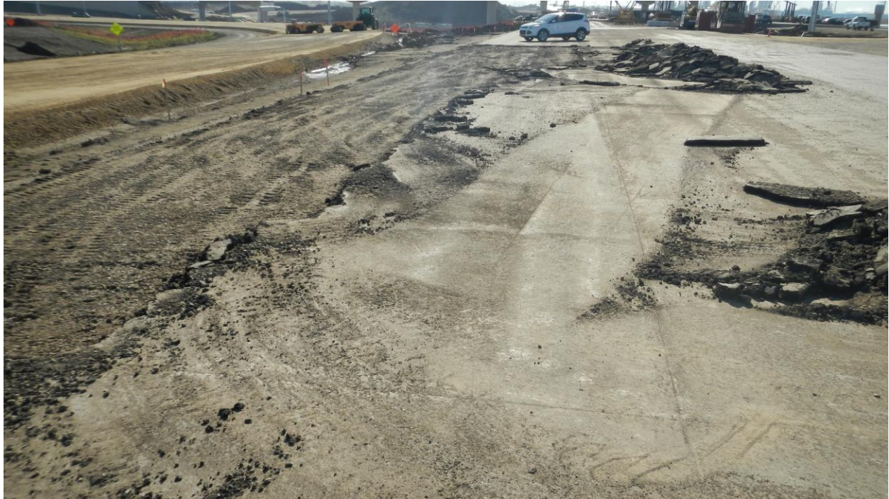
Figure 6: Extent of Repair Works Due to Deficiencies in Subgrade Compaction
