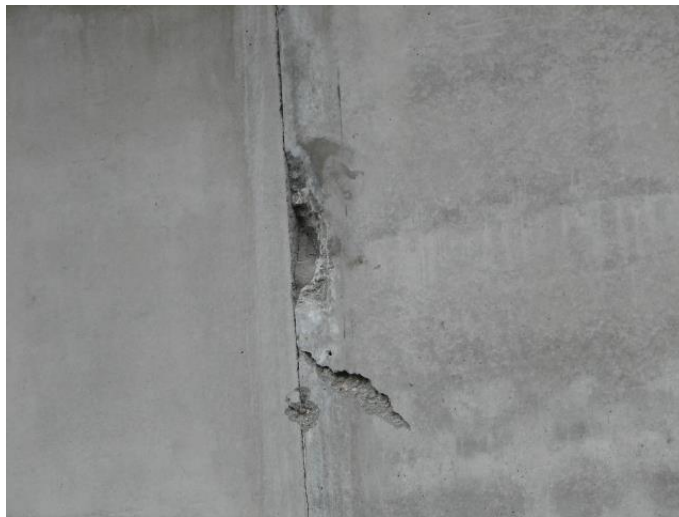
Figure 3: Spall Extension due to Incorrect Repair
