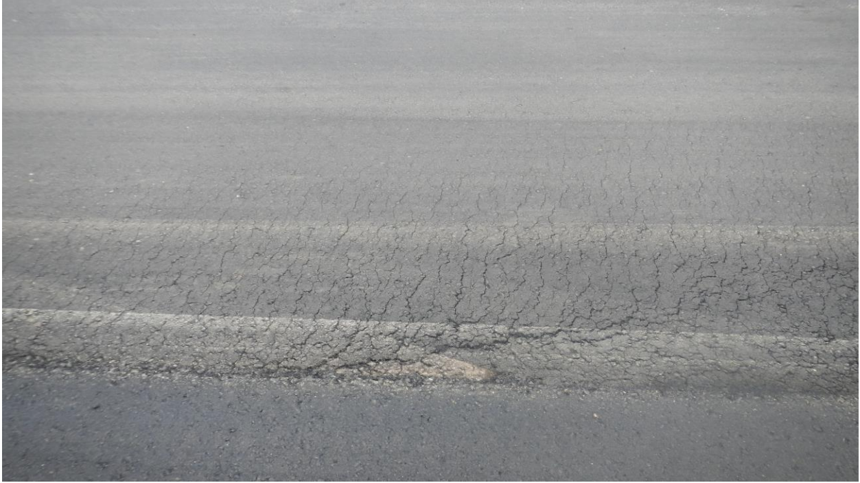
Figure 4: Surface Cracking and Differential Settlement on a Roadway
