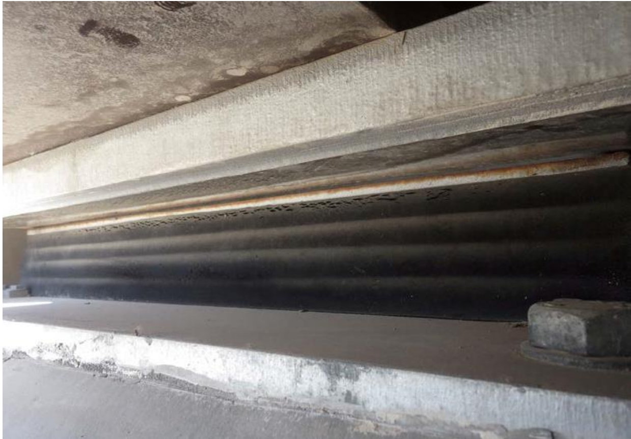
Figure 8: Failure of Elastomeric Bearing Pad with Bulging and Cracking before the End of Service Life
