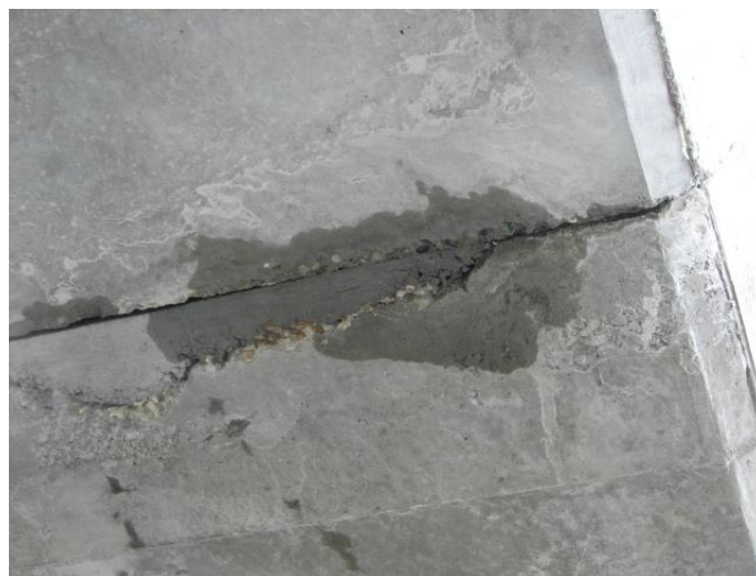
Figure 1: Improper Repair of Concrete Spall
