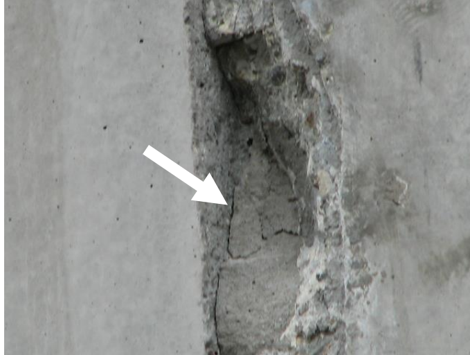
Figure 2: Spall at the Repair Location due to Incorrect Repair Method and Lack of Bonding as Pointed
