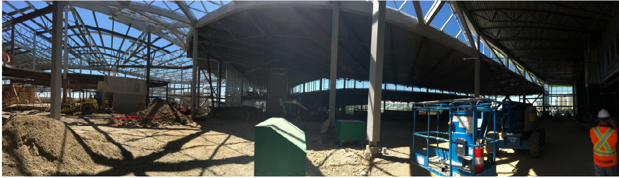
Figure 1 : Landscape photo of SRF to show the complex geometry of the building (Photo taken by Maxime S. Harvey from Canam group)
