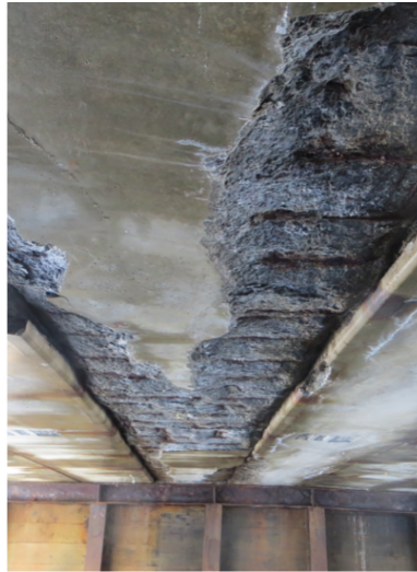
Figure 1. The Deterioration of the Case Study Bridge
