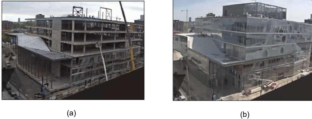
Figure 1: Isometric views of the MDE building a) at bare-frame stage; b) at full-frame stage (Bonne 2018)
