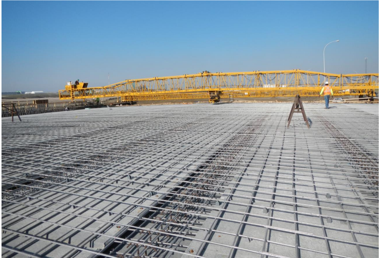
Figure 9: Rebar Connecting Precast Panels and Cast-in-situ Concrete Deck for a Monolithic Concrete Deck
