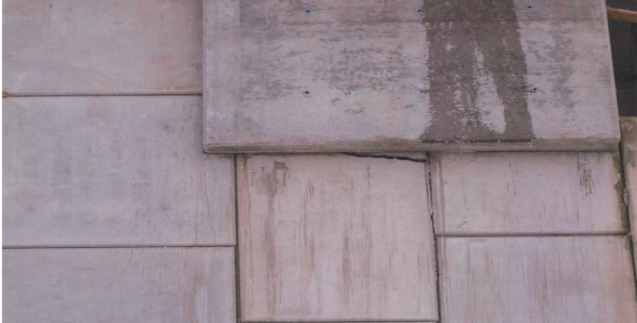
Figure 5: Cracks in MSE Wall Panels
