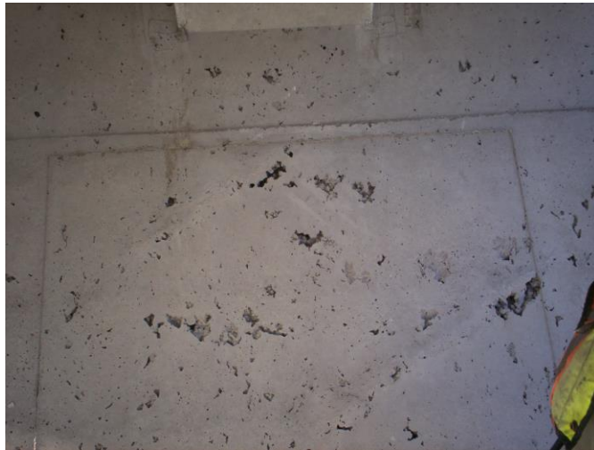
Figure 1: Honeycomb in Cast-in-place Concrete
