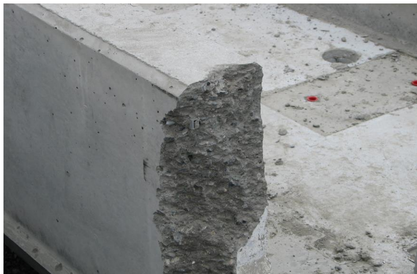
Figure 2: Corner Spall in Concrete Road Barrier
