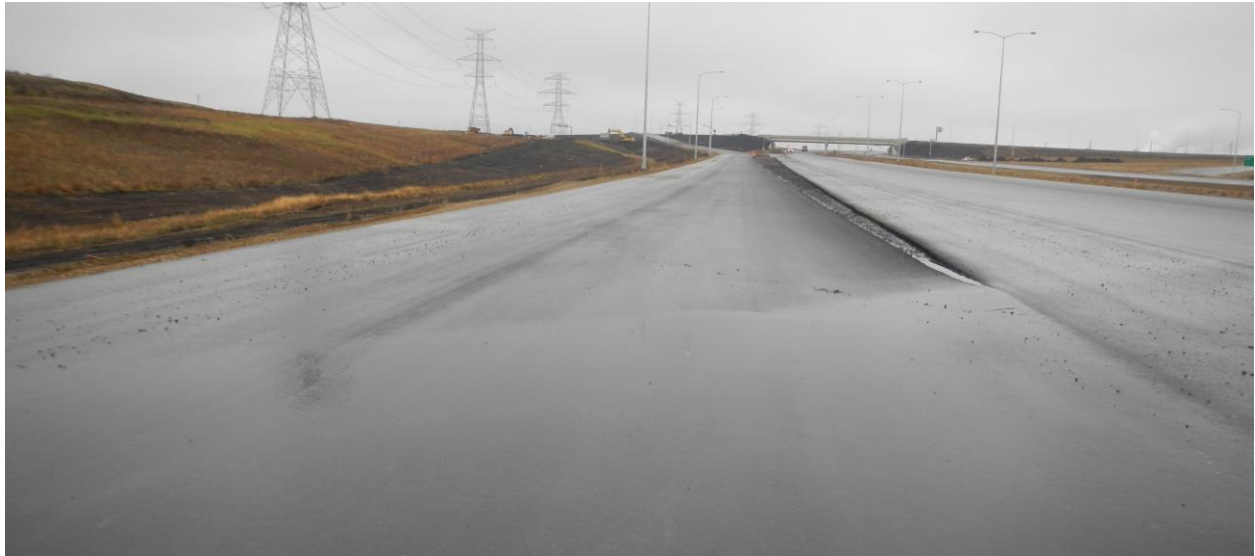
Figure 7: Roadway Settlement Due to Deficiencies in Subgrade Compaction
