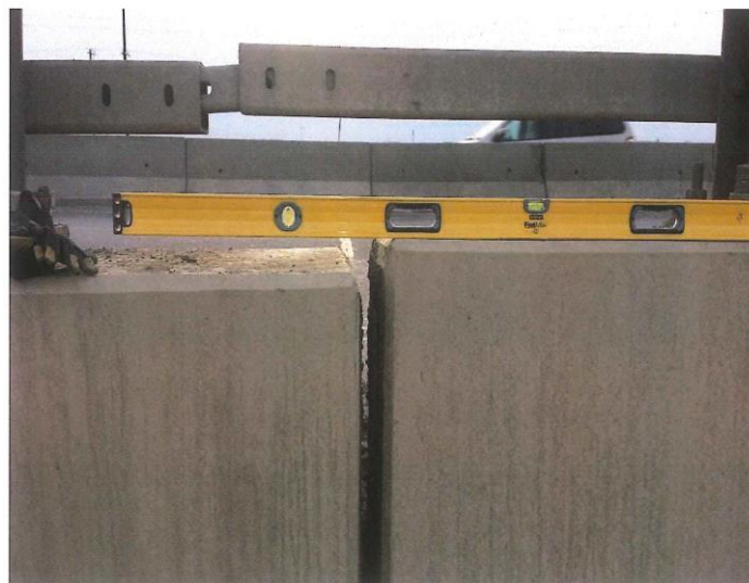
Figure 6: Approach Settlement Due to Deficiencies in MSE Wall Backfill Compaction
