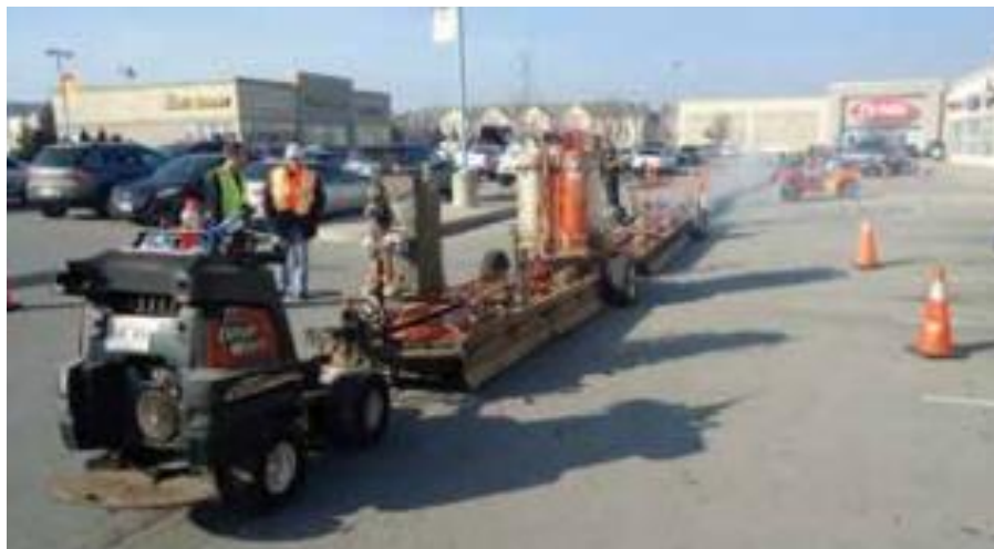
Figure 4: Infrared Heating Train (Heat Design Equipment Inc., 2017)
