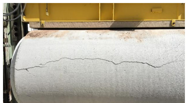
Figure 5: Double circular cage longitudinal cracking
