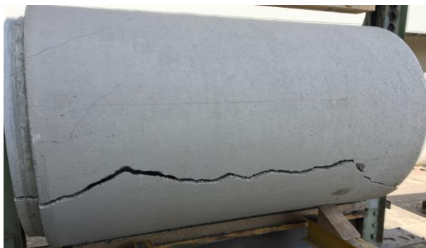
Figure 4: Single elliptical cage longitudinal cracking
