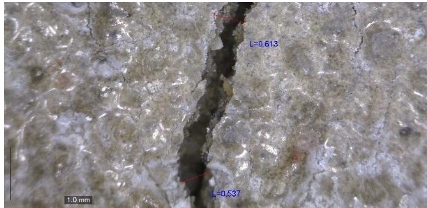
Figure 4: Typical plastic shrinkage crack observed under a microscope
