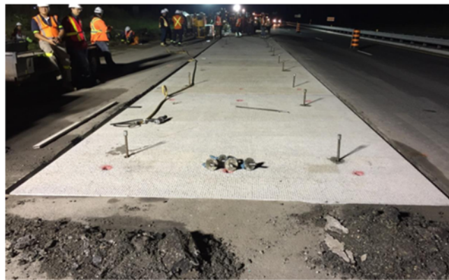
Figure 1: Precast concrete inlay panel installation in third lane of highway (Pickel and Tighe 2017)
