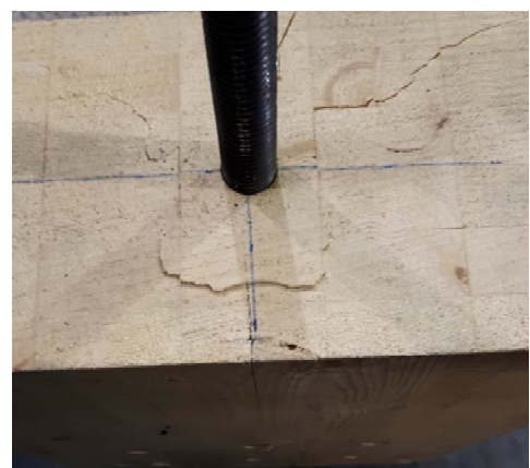
(c) Rod pull-out shearing along carved out hole edges with 45 degree cracks
