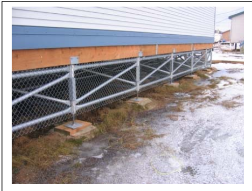
Figure 7: Multiple support pads and frame to building connections.
