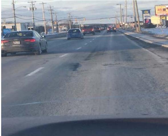
(a) Structural rutting
