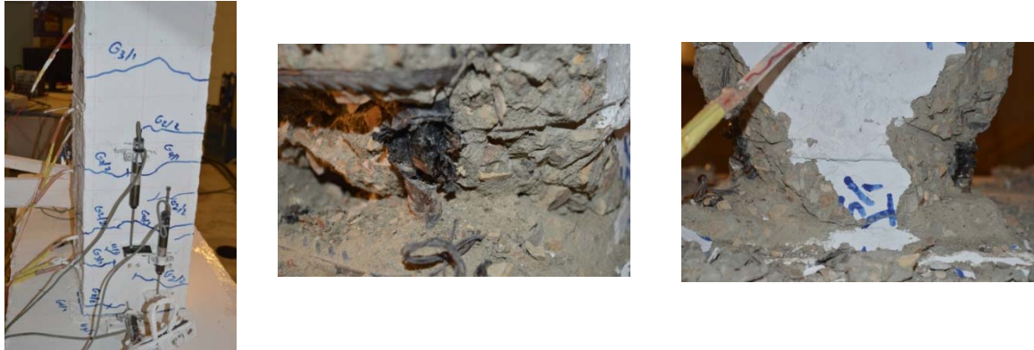
Figure 5: Failure mode of specimen F15
