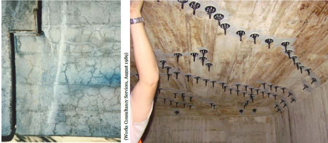
Figure 5: ASR Cracking to Half-Joint (left), ASR Cracking to Deck Soffit (right)
