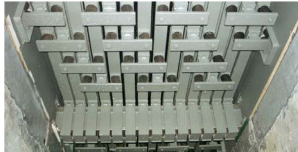
Figure 4: An installed Tensa-Modular expansion joint, viewed from below
