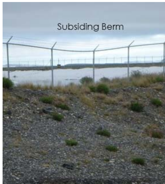
Figure 2: Forty centimetre subsidence in Kugluktuk sewage lagoon berm.
