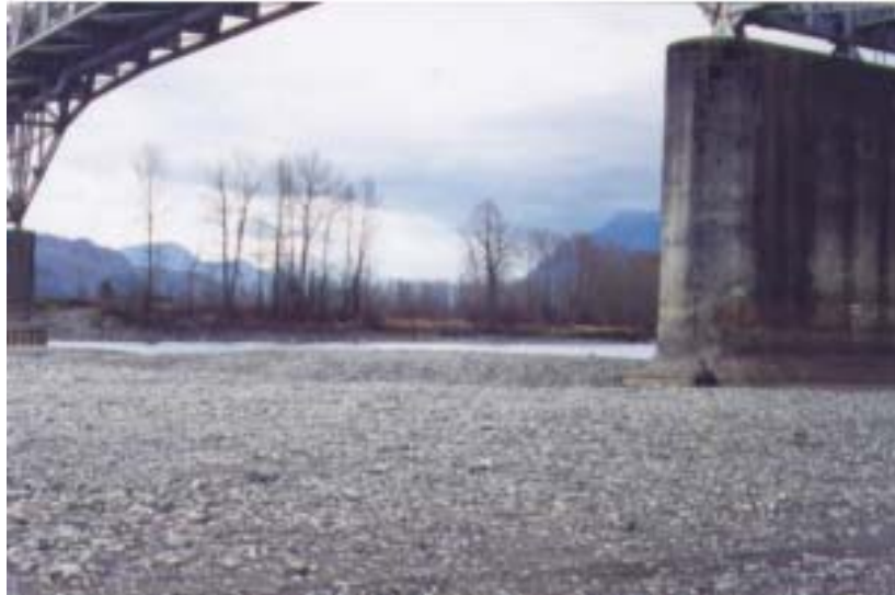
Figure 1: Scour hole downstream of a pier at Agassiz Bridge, Fraser River, BC.
