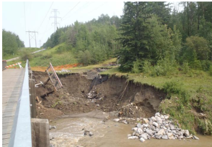
Figure 3: Damage caused to Whitemud Creek bank during 2012 overflow event (Photo courtesy of Paul Lach, City of Edmonton)
