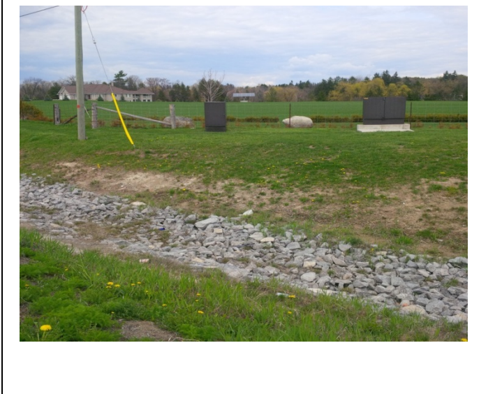
Figure 5: OPI & CPS equipment on concrete foundation
