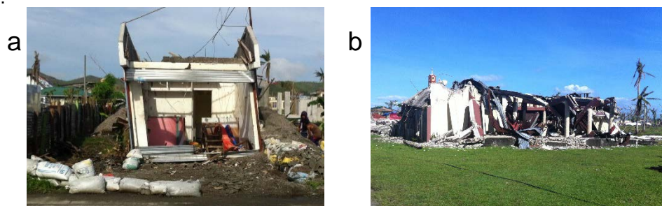
Figure 7: Small reinforced concrete buildings damaged by typhoon Haiyan.
