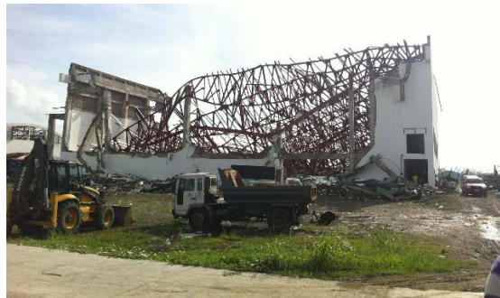
Figure 9. Large volume, newer reinforced concrete building with extensive damage.
