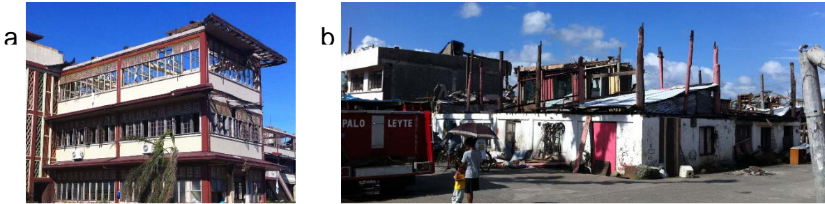
Figure 5: Older structures of timber construction with damaged secondary (cladding/roof) systems.
