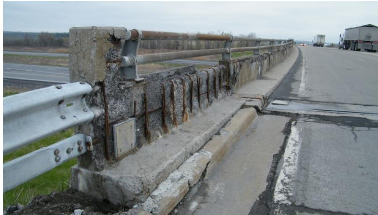
Figure 1: Corrosion of steel reinforcement in bridge guardrails
