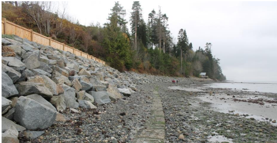
Figure 1: Example of hard shoreline armouring: armour rock revetment, Town of Qualicum Beach, BC
