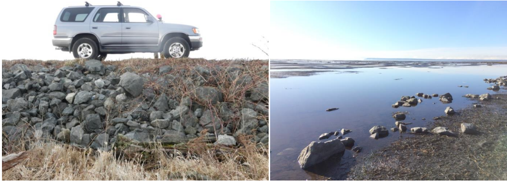
Figure 6: The pre-existing riprap revetment in poor condition (left), and riprap pieces in WMA post storm (right), Boundary Bay, Corporation of Delta, BC
