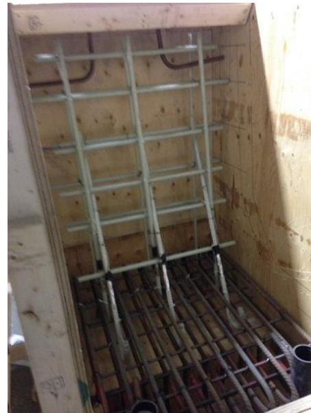
Figure 6: View of internal reinforcement in tested barrier specimen B-2
