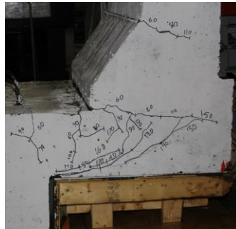
Figure 16: Crack on right side of B-3
