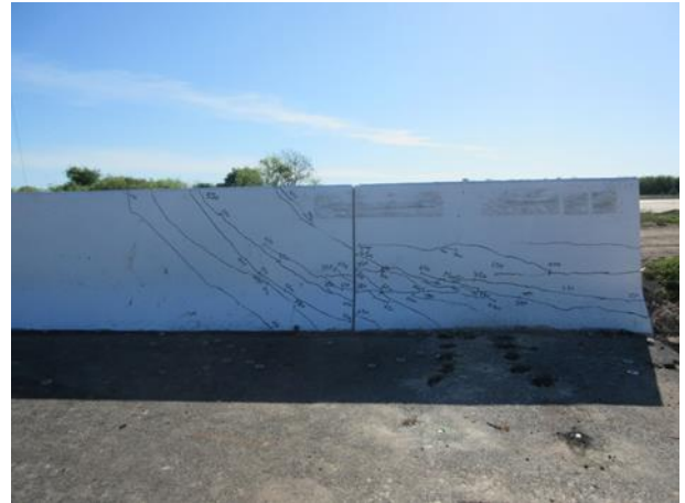
Figure 22: View of the crack pattern at the front face of the barrier wall at exterior location
