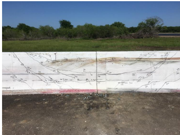
Figure 16: Front view of the flexural crack pattern and punching shear failure of the barrier interior location
