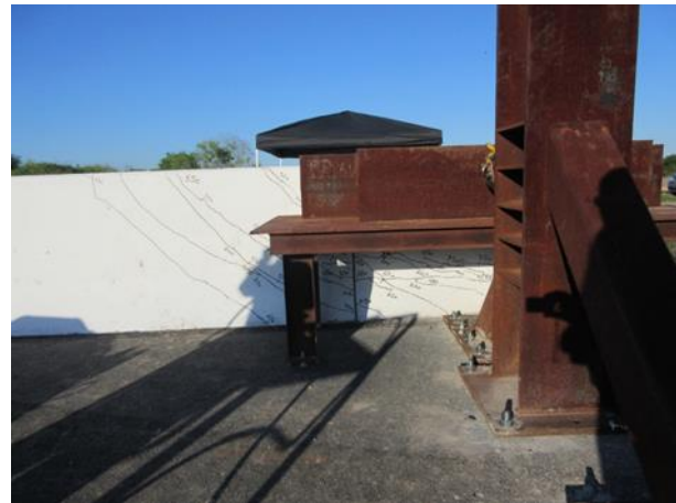
Figure 20: View of the horizontal flexural cracks within the loaded length, extending diagonally beyond the loaded length
