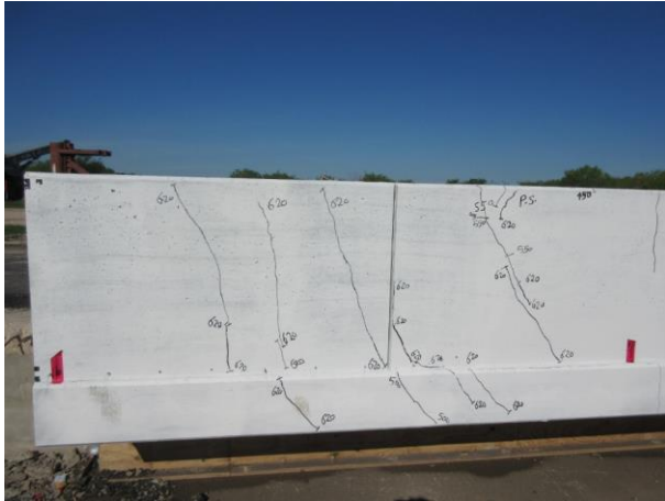
Figure 21: View of diagonal cracks at the back face of the barrier wall
