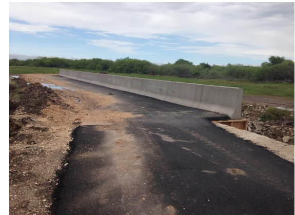
Figure 7: View of the barrier wall after removing the formwork and asphalt paving
