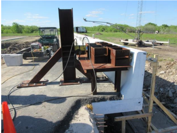
Figure 9: View of the loading setup for the static load test at exterior location of the barrier wall
