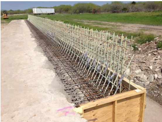
Figure 5: View of GFRP and steel bar arrangement at the beginning of the constructed barrier-deck system
