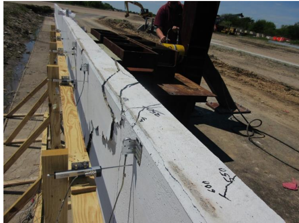
Figure 14: View of the punching shear crack at the top of the barrier wall, extending to the back of the wall at failure
