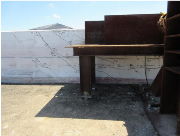
Figure 13: View of the horizontal cracks within the loaded length of the barrier, extending diagonally outside outside the right side of the loaded length
