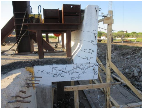
Figure 19: View of the crack pattern at the side of the barrier wall and slab cantilever at failure
