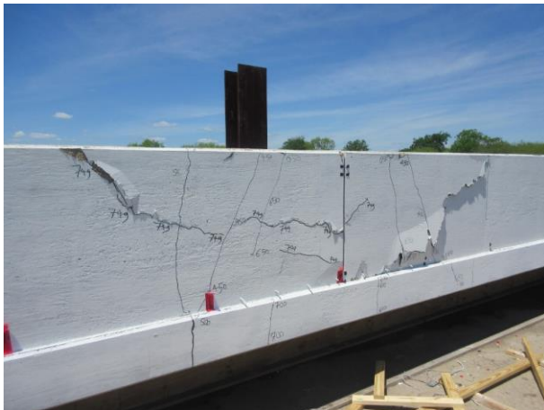
Figure 15: View of the punching shear failure at the back face of the barrier wall after removing the timber frame
