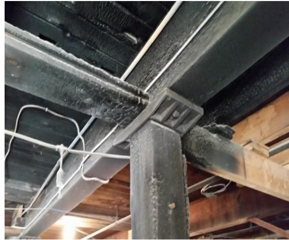
Figure 4. An arson attack on heritage timber where the smaller timber beam components had significant damage, whereas the larger column had minimal damage as the core cross-section remained (authors' photo).
