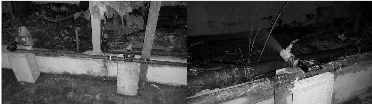
Figure 6: One-inch and Two-inch PVC Pipelines
