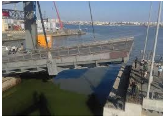
Figure 13: Cold test of Movable bridge bay
