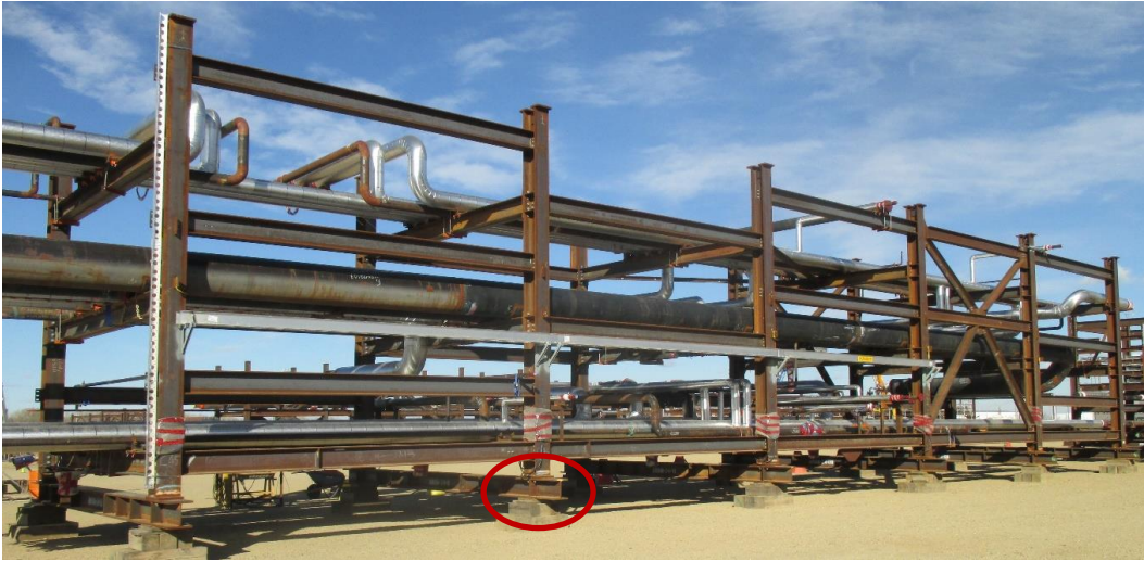
Figure 1: A module sitting on blocks ready to be shipped for site installation (reprinted with permission from PCL Construction Inc., 2016)
