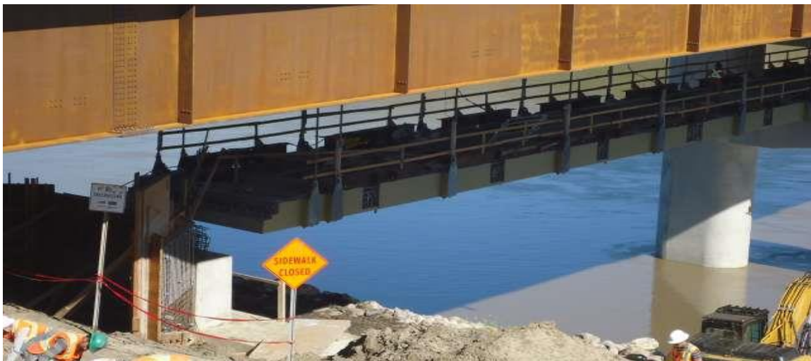
Figure 7: Steel Girder Bridges Crossing North Saskatchewan River during Construction (above) and the Under-slung Pedestrian Bridge (below)
