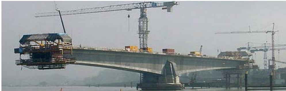
Figure 1: Construction of the Pierre Pflimlin bridge using the balanced cantilever method (Leonard, 2007).
