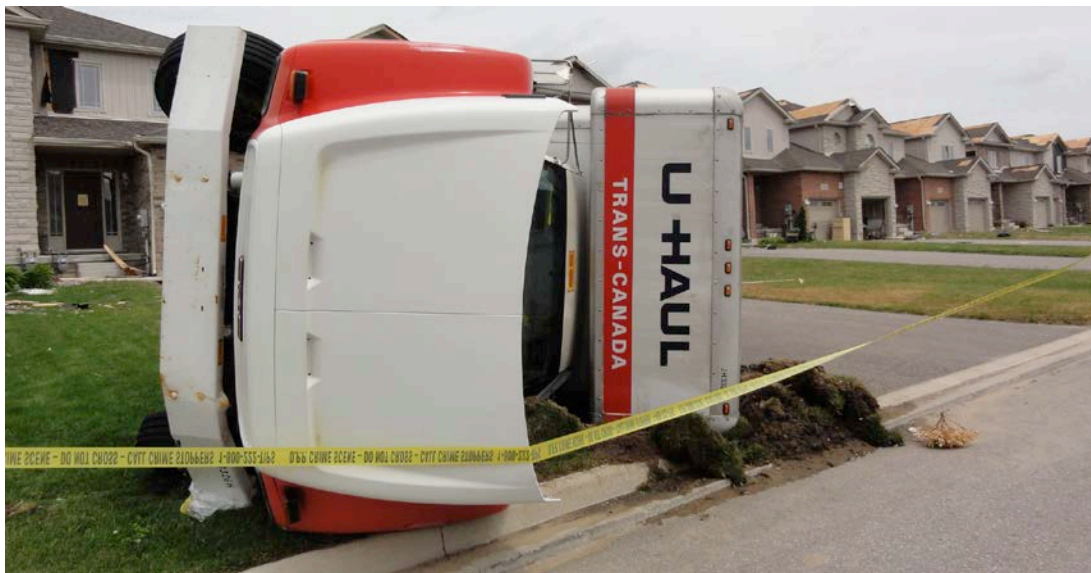
Figure 7. Overturned U-Haul truck in the foreground with repetitive shingle, roof sheathing and garage door failures on houses on Banting Cres. in the background.
