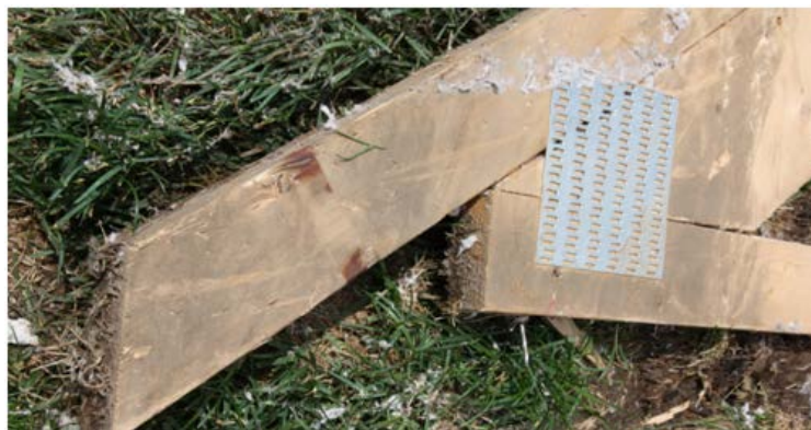
Figure 4. Roof truss from a house on Stonemount Cres. This roof truss had only 1 toe-nail in the connection, rather than the code-required 3.
