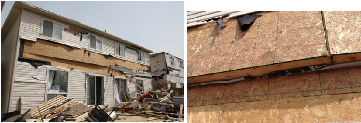
Figure 6. Wall failure due to missing inter-storey connections.
