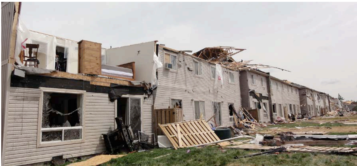
Figure 5. House with observed roof and wall failure. The second story of this house has been blown open. The connections have come apart and the wall has been fallen nearby.
