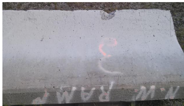
Figure 2: Low Deteriorated Barrier
