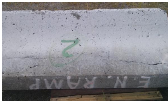
Figure 1: High Deteriorated Barrier
