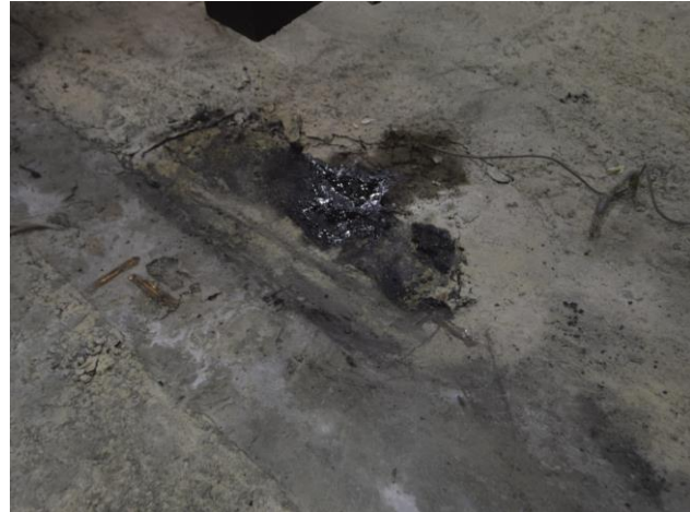
b. Close-up view for the punching shear failure at the wheel footprint
