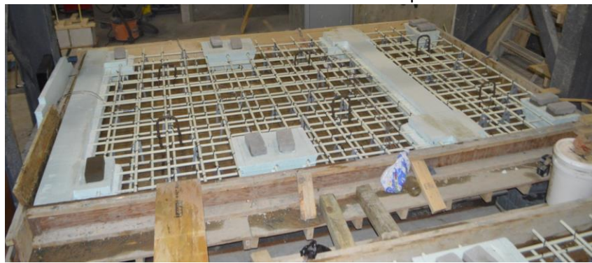
c. View of GFRP bars and Styrofoam to form the connection Figure 3. Construction of the precast FDDP with C-shape connection
