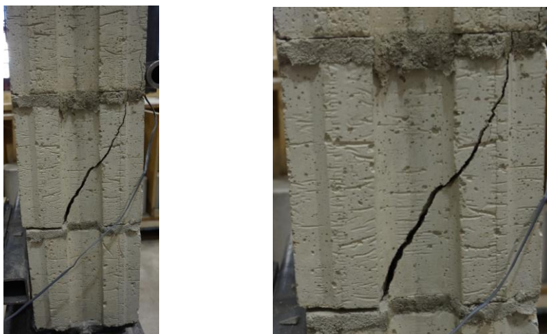
Figure 8: Typical combined sliding shear and diagonal tension shear failure (Specimen F1)
