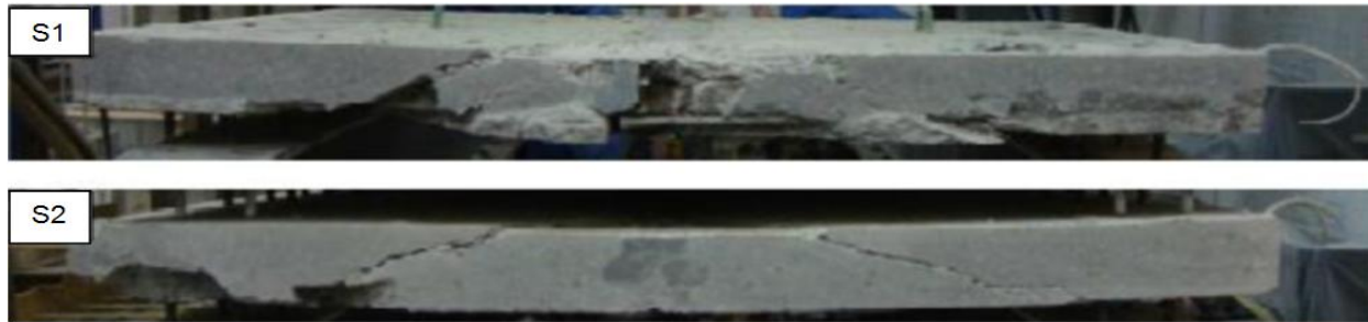
Figure 10 Views of saw-cut slab segments after punching shear failure for deck slabs S1 and S2
