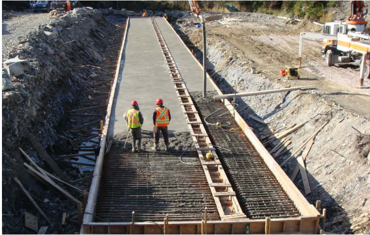
Figure 12. Site casting two parallel 1.250 x 5.350 m -70m long footings complete with keyway for Arch placement.
