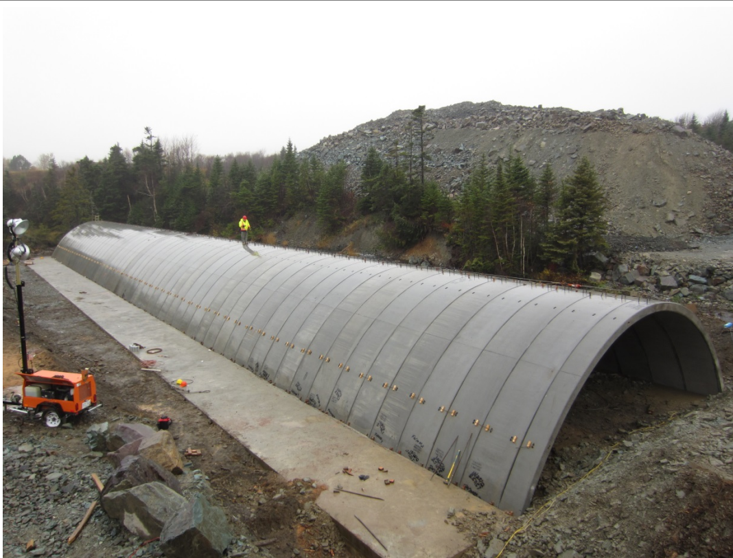
Figure 17. Arch element erection is complete. Grouting of footing keyway, casting of crown beams and placing filter fabric over joints is must be completed before backfilling.
