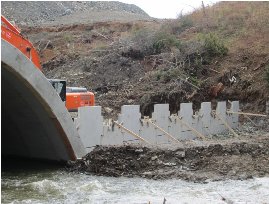
Figure 18. River is returned to natural alignment. Backfilling of headwalls and wing walls begins
