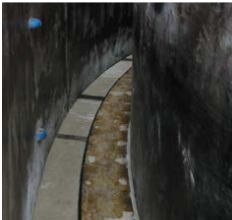
Figure 7. Steel forms are set to the design curve by matching the template.
