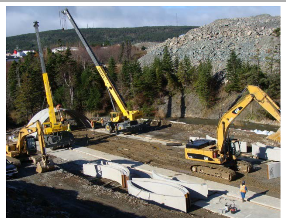
Figure 14. Two cranes place the first two elements. After placing 4 elements work can proceed with one crane and the second crane can be released.
