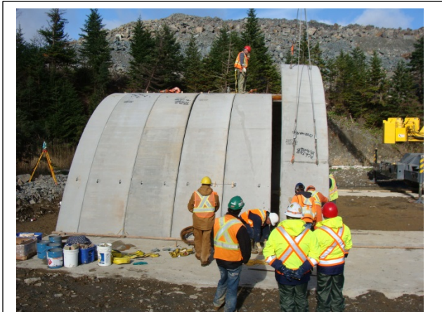
Figure 15. Rigging is pre-set to place the element at the 1.4% down grade slope.
