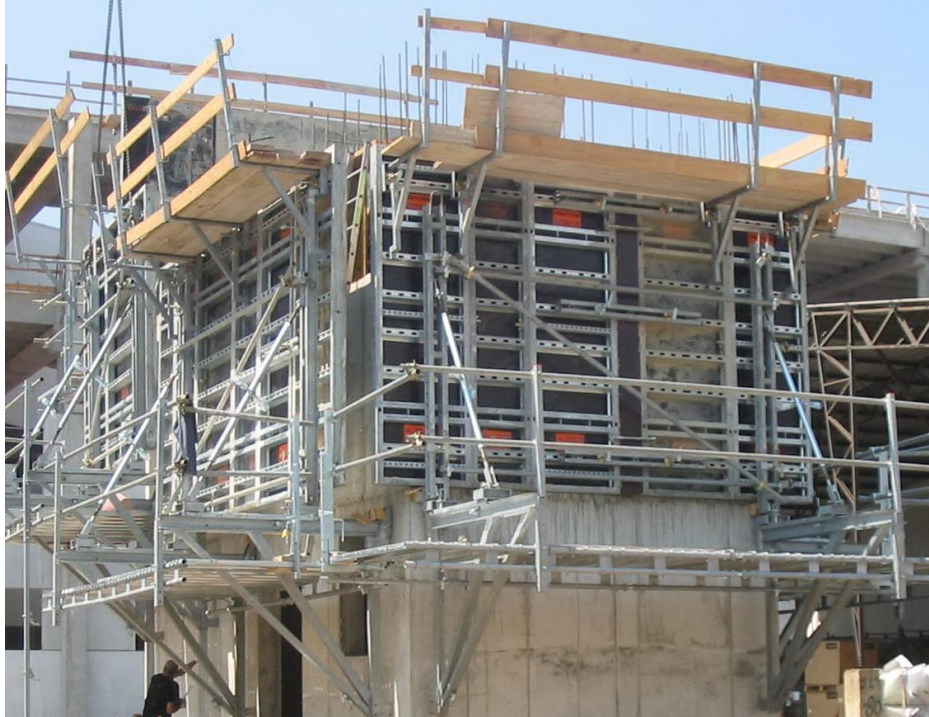
Figure 1: Lifting a jump form (photo taken and authorized for reuse by (Destil, 2008))
